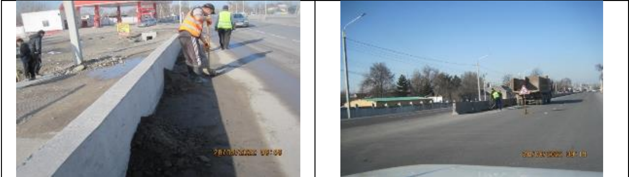
Figure 28 Cleaning of area near parapets from earth waste and removal of waste from the road
