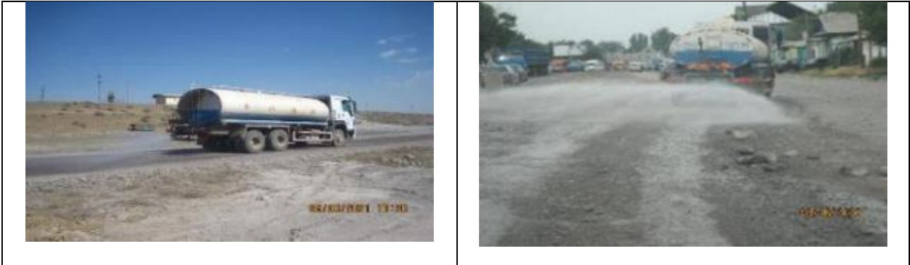
Figure 27 Water sprinkling works. Road to the production site and at the road construction site in the Voенno-Antonovka
