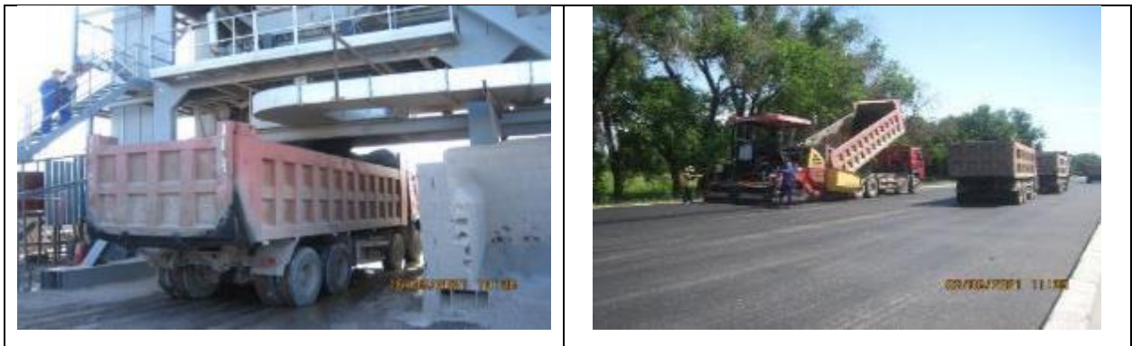
Figure 23 Loading of asphalt mixture into dump trucks and unloading into asphalt pavers.
