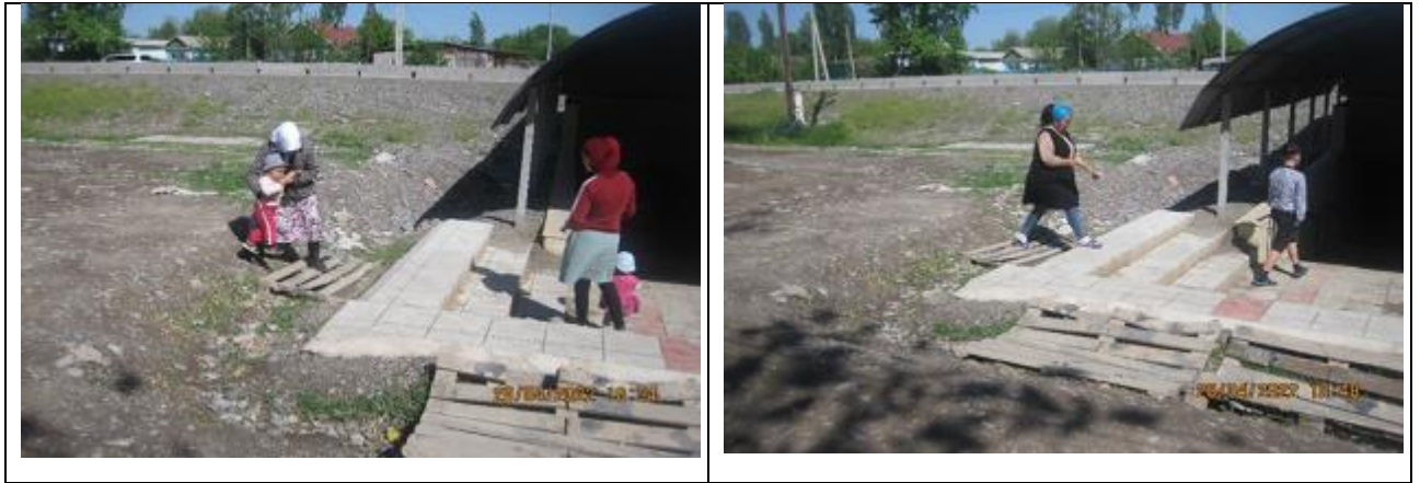
Figure 33 Violations near the underpass located opposite the school in the village of Novonikolaevka
