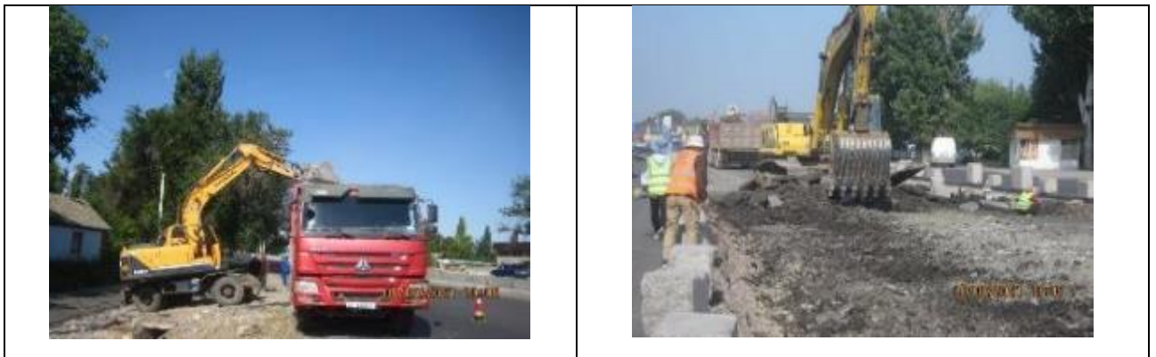
Figure 55 Taking out of the removed asphalt in the village of Voенно - Antonovka.
