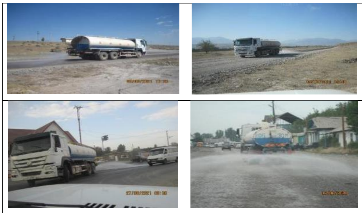
Figure 16 Dust suppression (water sprinkling). The road to the production site and at the road construction site
