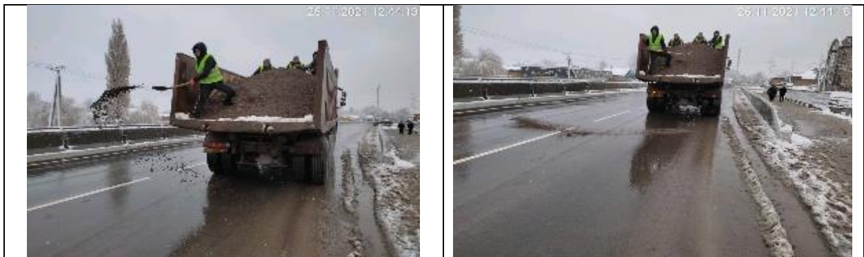
Figure 26 Spreading sand on the road. ilce control.
