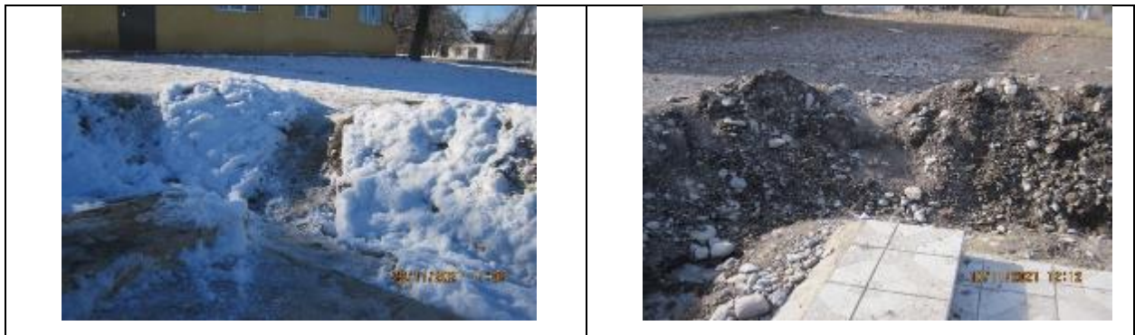
Figure 32 Construction waste around the underpass located near the school in the village of Novonikolaevka.
