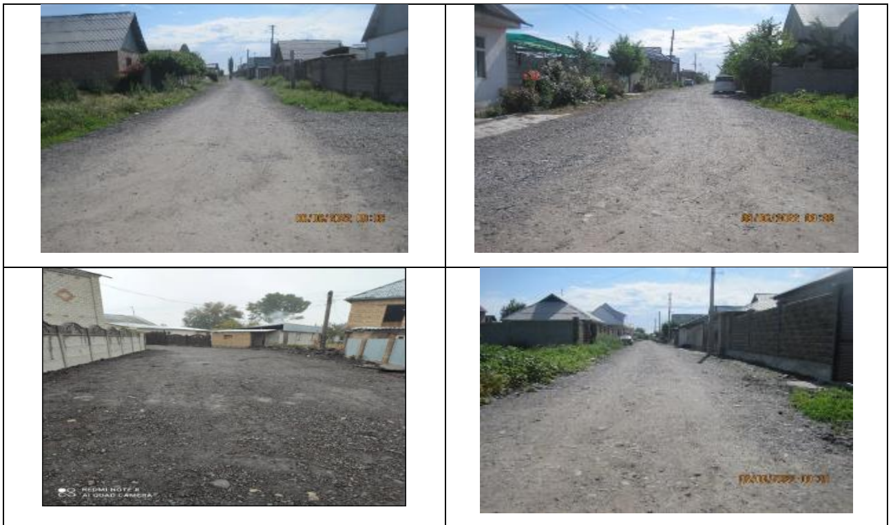
Figure 56 Backfilling of old asphalt on internal roads in the village of Voенно – Antoovka
